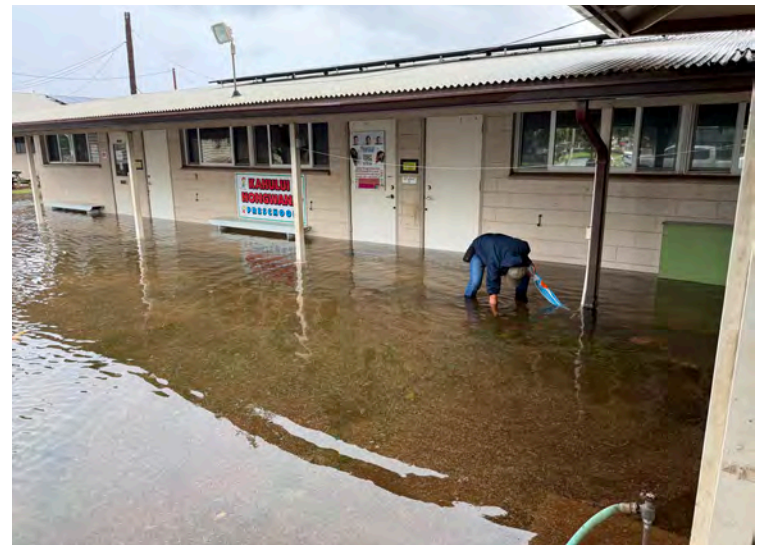
Doug Toyama works to clear a drain as floodwaters begin receding at Kahului Hongwanji Preschool.
